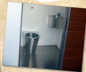
Stainless steel toilet
